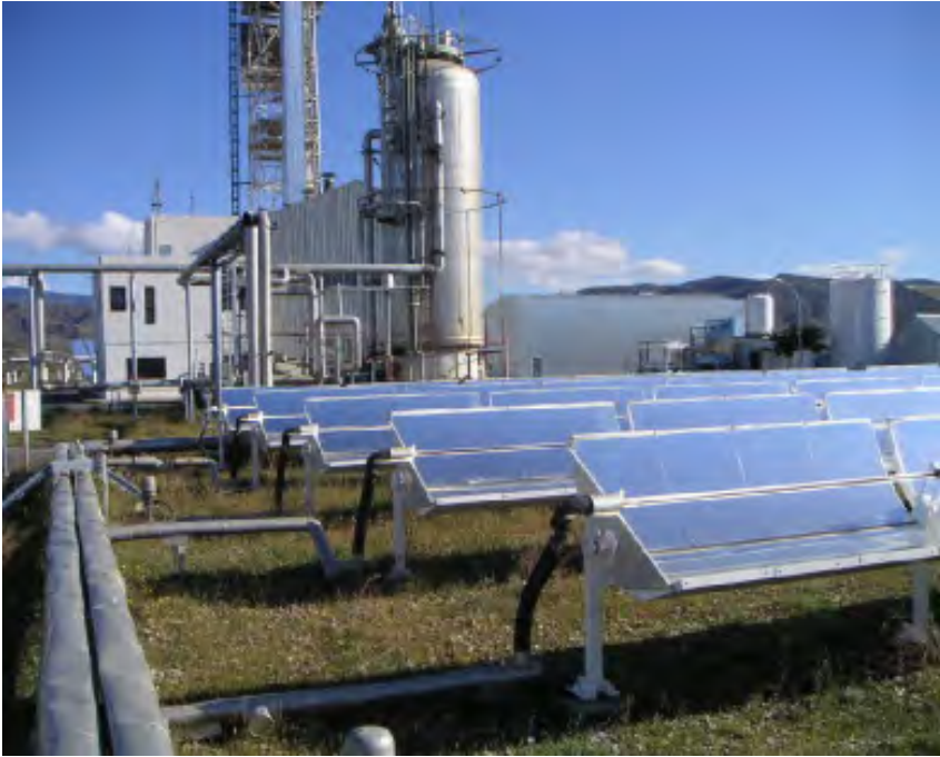
Figure 2.10: Acurex distributed collector system at the Solar Platform of Almería (PSA), Spain.
